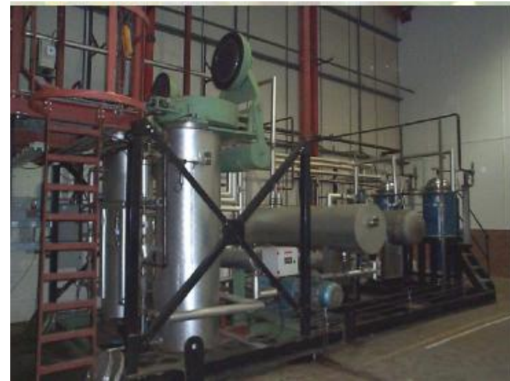
2x400 litre SCO 2 Extraction Plant
